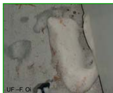
termite frass in foam.
