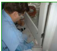
Foam treatment for drywood termites in a door.
